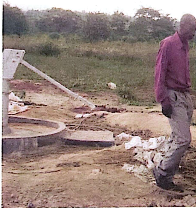
Non-functional. A man walks past a disfunctional borehole in Bujaaja village, Mpasana Sub-county recently. PHOTO BY ALEX TUMUHIMBISE.
