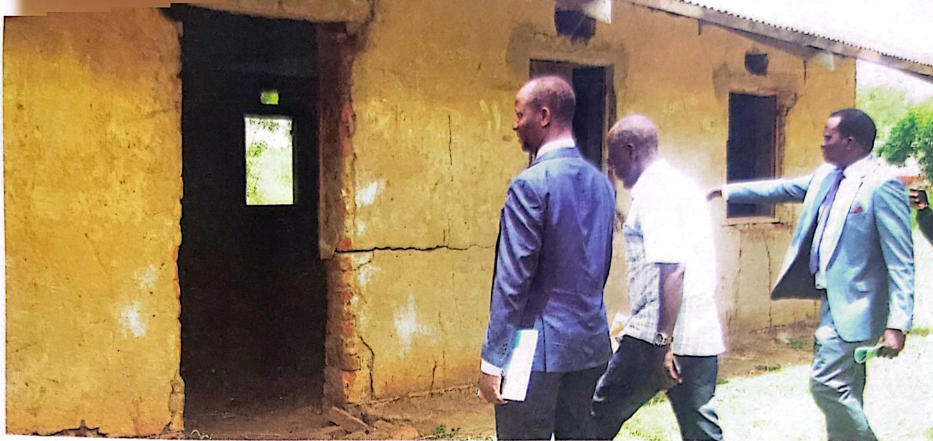
On the ground. MPs Ibrahim Semuju Nganda (left), Hassan Kaps Fungaroo (right) and Ogoko Sub-county councillor Hassan Manzu inspect one of the dilapidated classrooms at the institute last Friday. PHOTO BY FELIX W OKELLO
