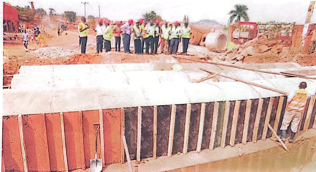
Engineers from the works ministry and Makindye municipality inspecting the works on Namasuba-Ndejje-Kitiko road on Tuesday. Photo by Job Nantakiika
