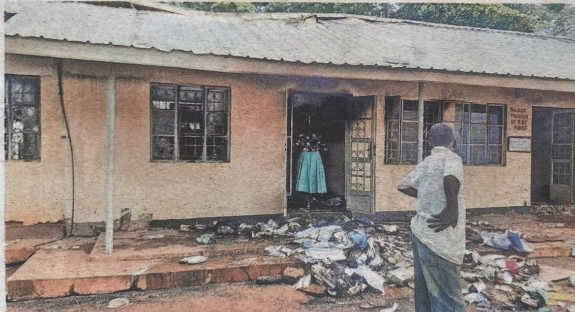
A resident and health worker inspect the burnt drug store at Bulumbi Health Centre III last Wednesday. PHOTO/DAVID AWORI
