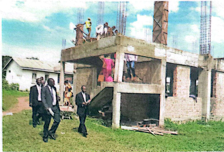
The Director General for Health Services, Dr Henry Mwebesa (Right), on a tour of a 400-bed ward under construction at Luweero Health Centre IV last month. PHOTO BY DAN WANDERA
