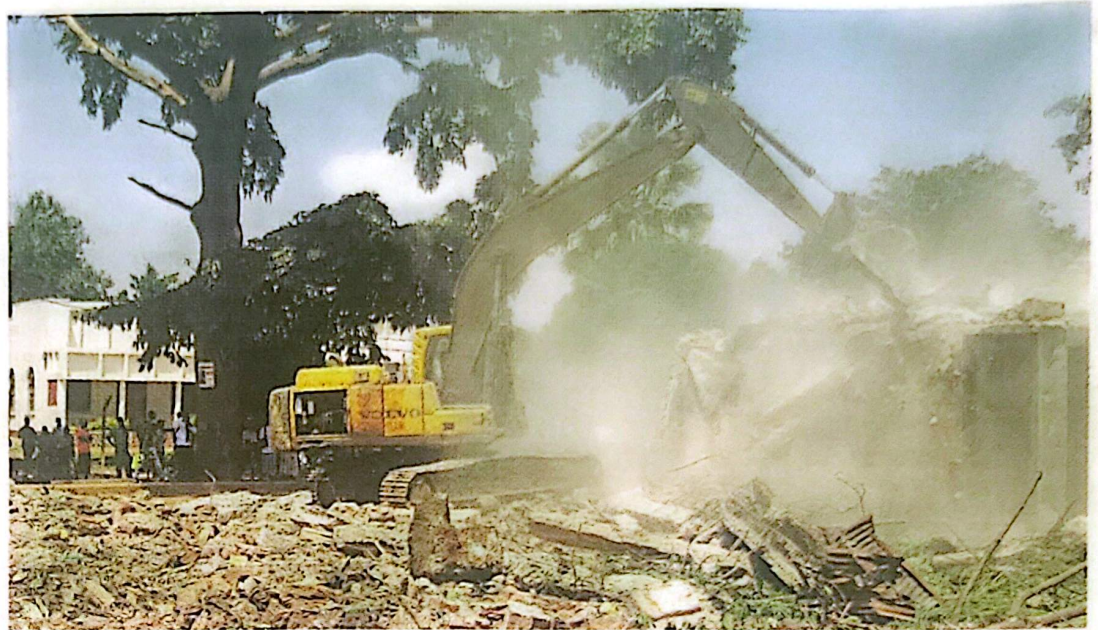
St Luke House that was demolished at the request of the owner.
