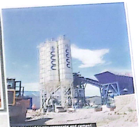
The silo used to mix aggregate and cement
