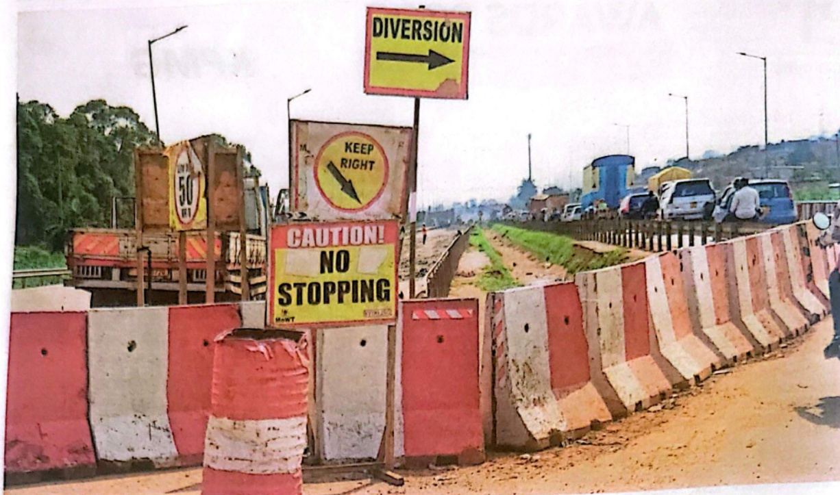
Drivers should stay alert to unusual roadside activity, obstacles, or irregular traffic patterns. PHOTO/MICHAEL KAKUMIRIZI
