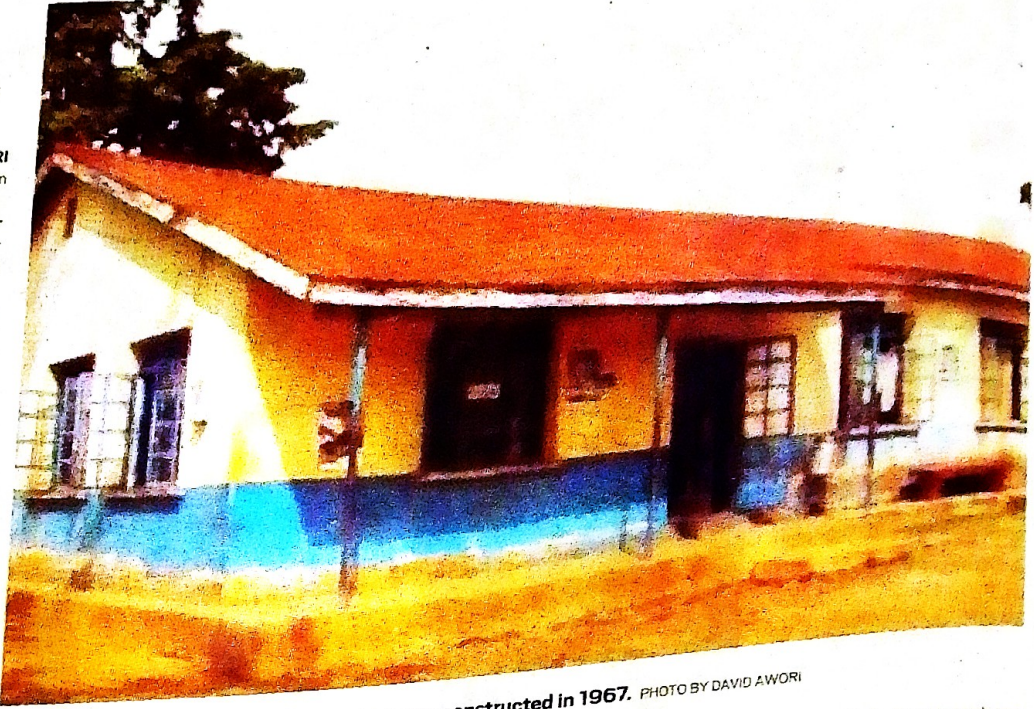
Dilapidated. Busitema Health Centre, which was constructed in 1967. PHOTO BY DAVID AWORI
