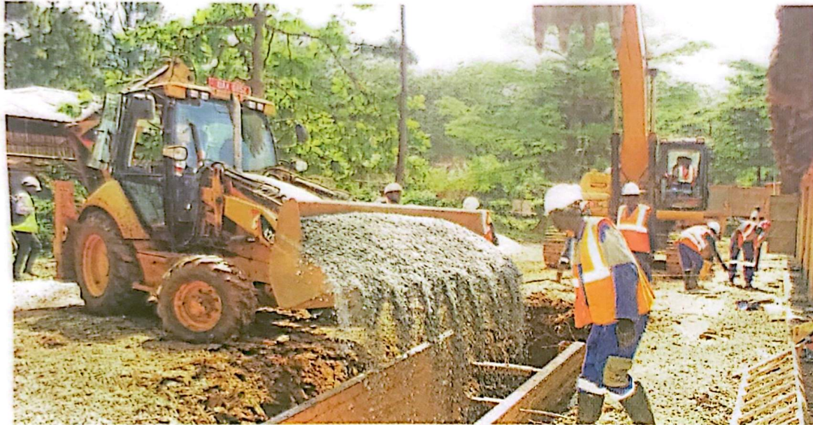
Sogea Satom engineers putting aggregates in one of the trenches at Centenary Park where they will be installing water pipes on Tuesday. Photo by Lawrence Mulondo
