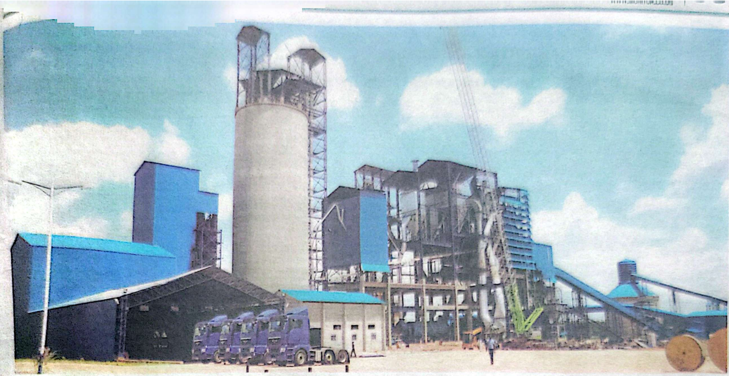
To use power. National Cement factory that is currently under construction in Tororo Municipality. COURTESY PHOTOS
