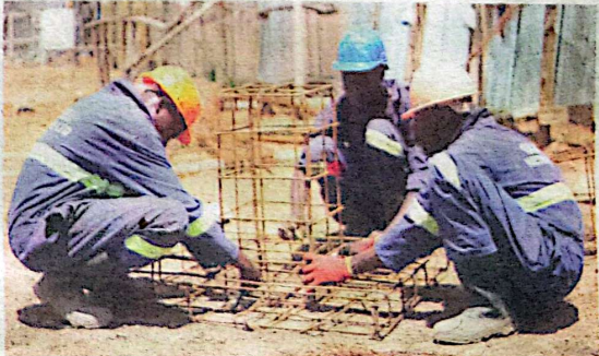
In progress. Workers doing civil works at Nyakesi substation in Tororo Municipality.
