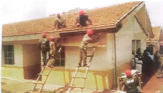
At work. The UPDF officers and the Rwandan military contingents renovate Tororo hospital at the weekend. PHOTO BY JOSEPH OMOLLO
