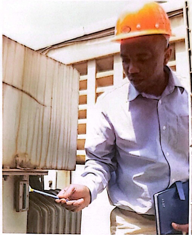
Segken Services Limited founder Mr Sotius Segawa explains the business operations at a control room for a transformer at Airtel House in Kampala. PHOTO BY GODFREY LUGAJU
