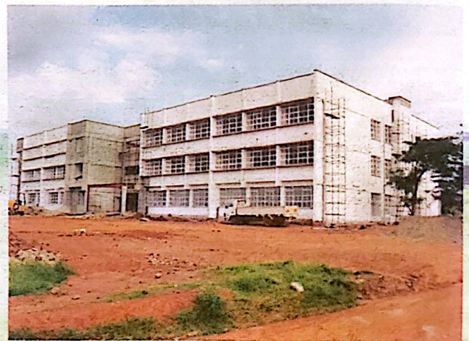
The ongoing construction of laboratory and lecture blocks for faculty of Engineering by PRISMA UG.Ltd
