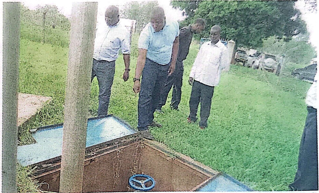
Kweronda (in blue T-shirt) and his team inspecting the metering system of Minakulu water project. Photo by Agnes Nantambi
