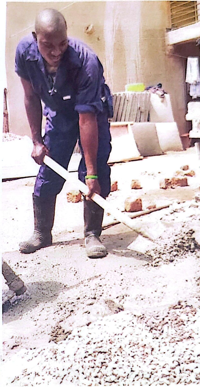
Constant inhaling of cement will lead to a number of ailments. But most of these can be prevented through taking precautions. NET PHOTO
